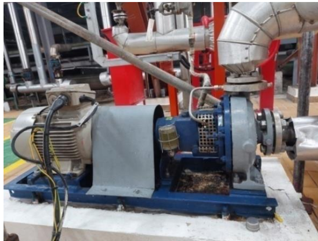
Figure 3. Pump motor 23P02
